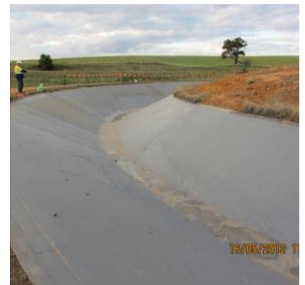
Figure 3. Open concrete water supply channel AFTER remediation with Geofabric and Elaston-W80 polyurea
