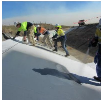
Figure 2. Open concrete water supply channel DURING remediation with Geofabric and Elaston-W80 polyurea
