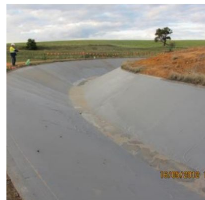
Figure 3. Open concrete water supply channel AFTER remediation with Geofabric and Elaston-W80 polyurea
