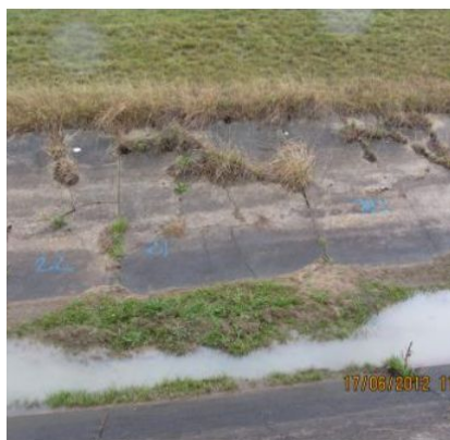
Figure 1. Open concrete water supply channel BEFORE remediation with Geofabric and Elaston-W80 polyurea
