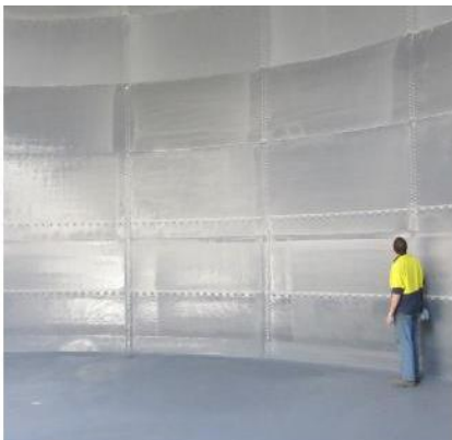
Figure 1. Steel panel tank used for community drinking water supply lined with Tufflon-P90.
